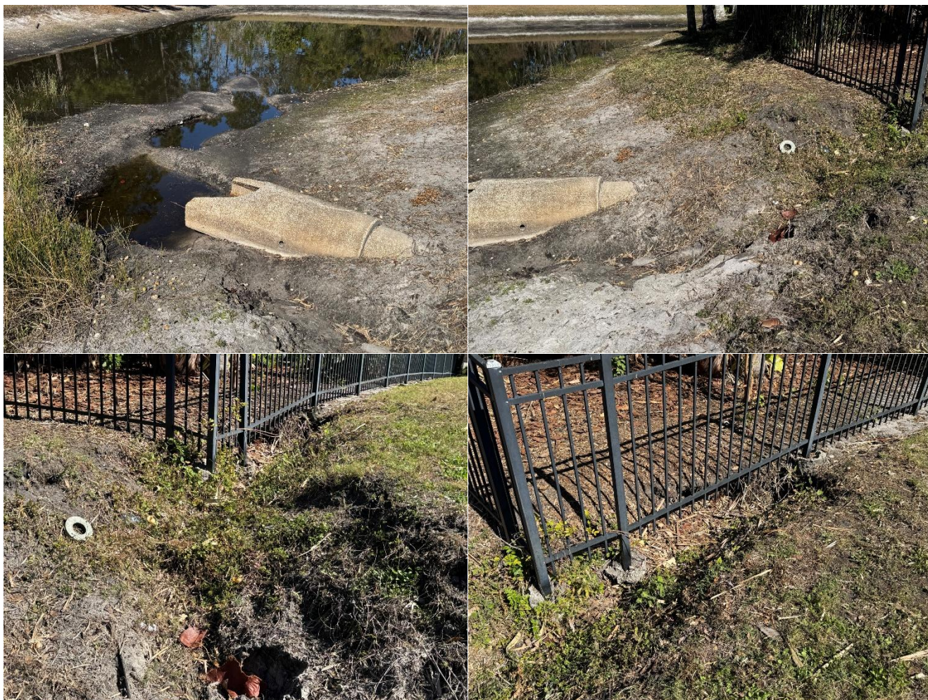
Photo 12 – Displays Pond 20 pond bank erosion around drain inlet. Erosion is affecting CDD and private property. Water source appears to come from resident irrigation.
