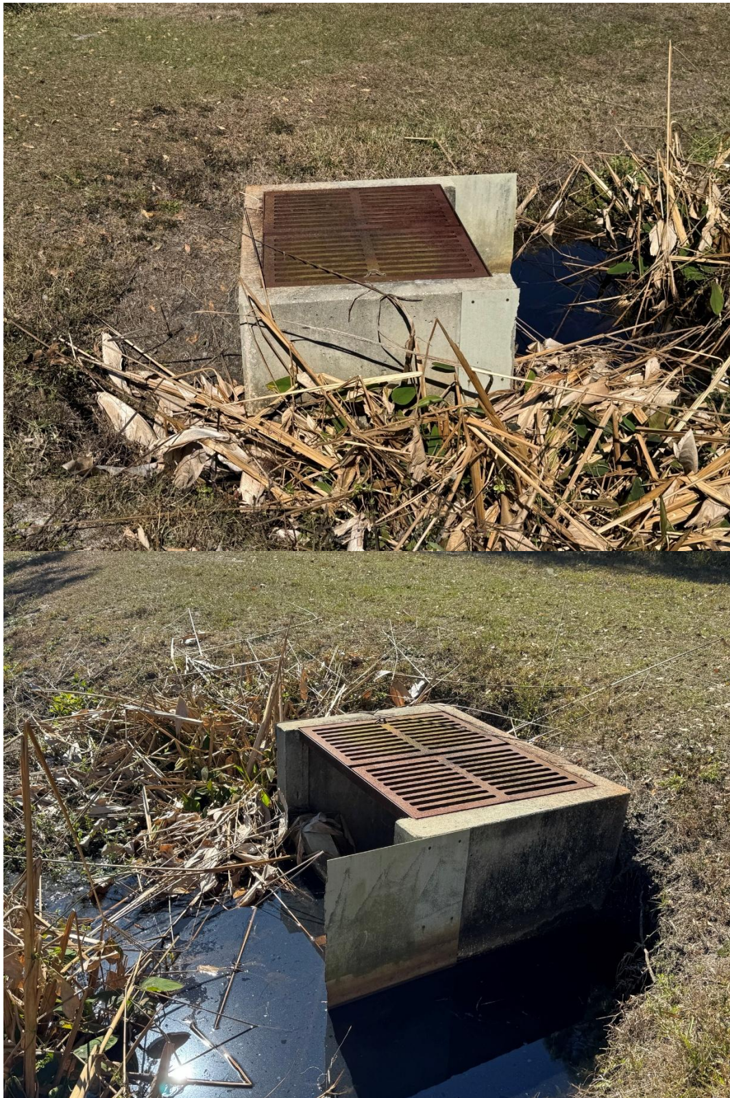
Photo 5 – Displays Pond 8 control structure with a broken skimmer and minor erosion on the back side of the structure. The pond equatic plants are greatly helping reduce erosional issues.
