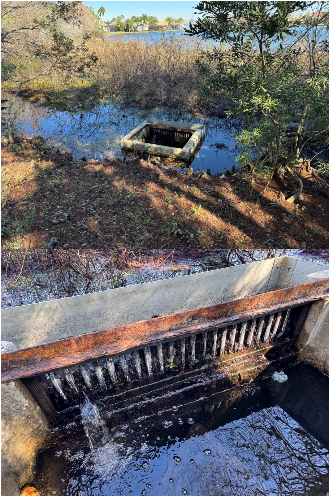
Photo 7 – Displays Pond 11 outfall control structures' clogged weir opening and displaced top grates. The two halves of the grate have fallen into the structure.
