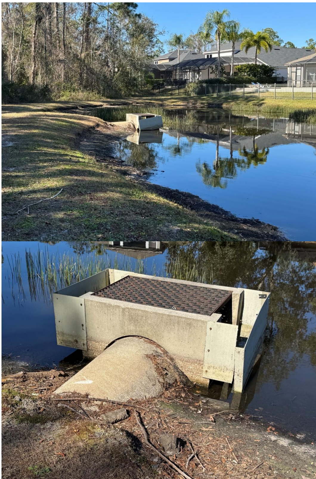
Photo 9 – Displays Pond 16 outfall control structure with the skimmer broken on one side. Structure pipe has experienced some erosion but it does not affect the operation of the structure.
