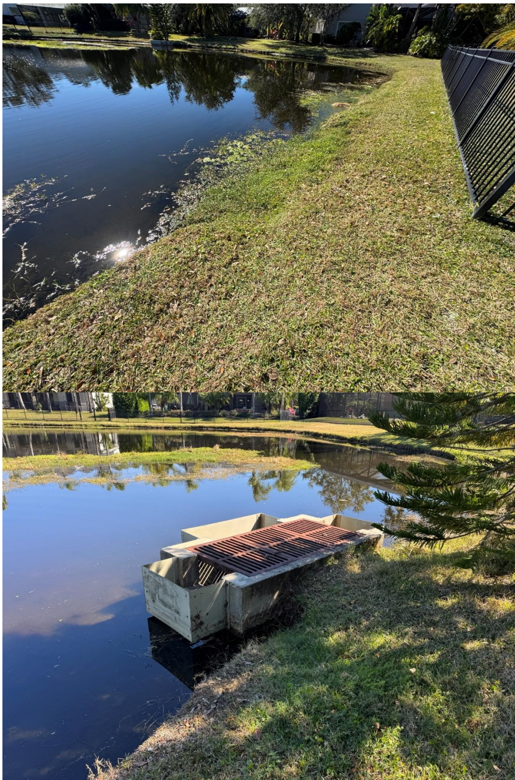
Photo 11 – Displays Pond 19 area of minor pond band erosion and minor erosion on the back side of the control structure.
