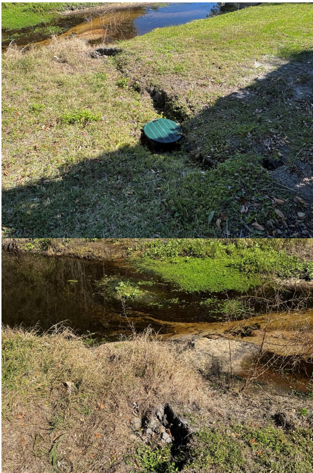
Photo 13 – Displays current condition of the erosion repair with catch basin at Double Branch Canal and Meridan Point Dr. Area around catch basin has eroded and erosional channel has formed. Sediment has deposited in Double Branch Canal.
