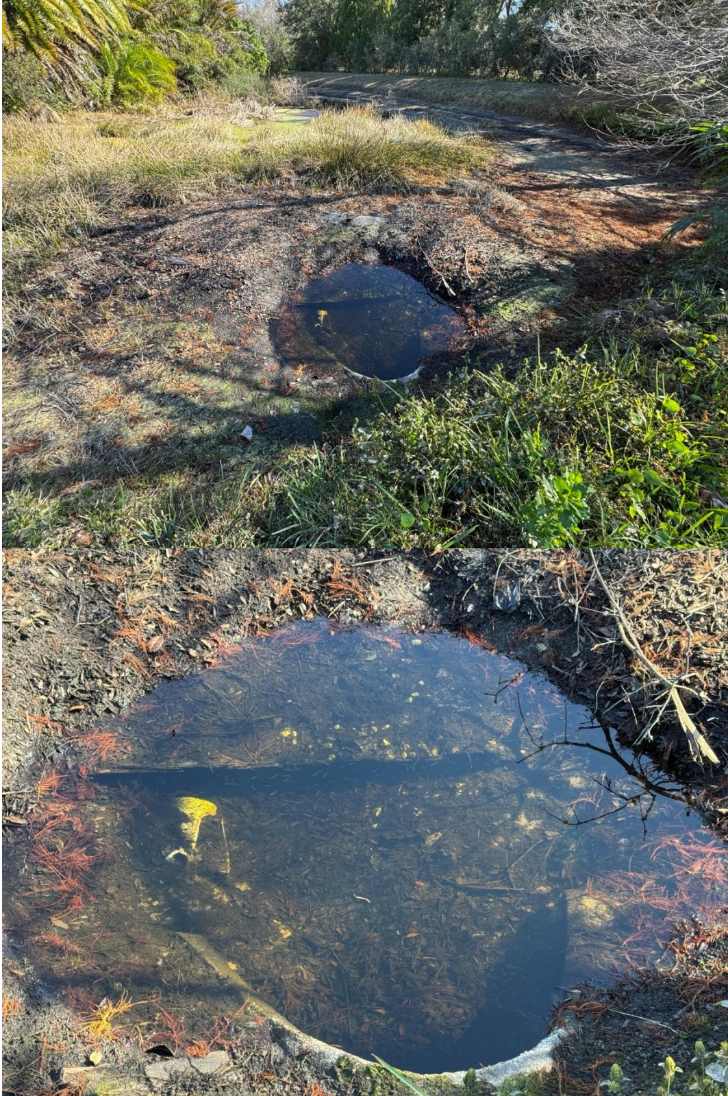
Photo 4 – Displays Pond 7 sediment build up at the drainage inlet. Silt build up does not appear to be impeding flow.
