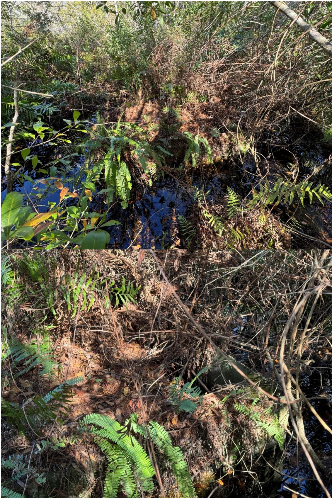
Photo 2 – Displays Pond 4 control structure overgrown and requires maintenance.
