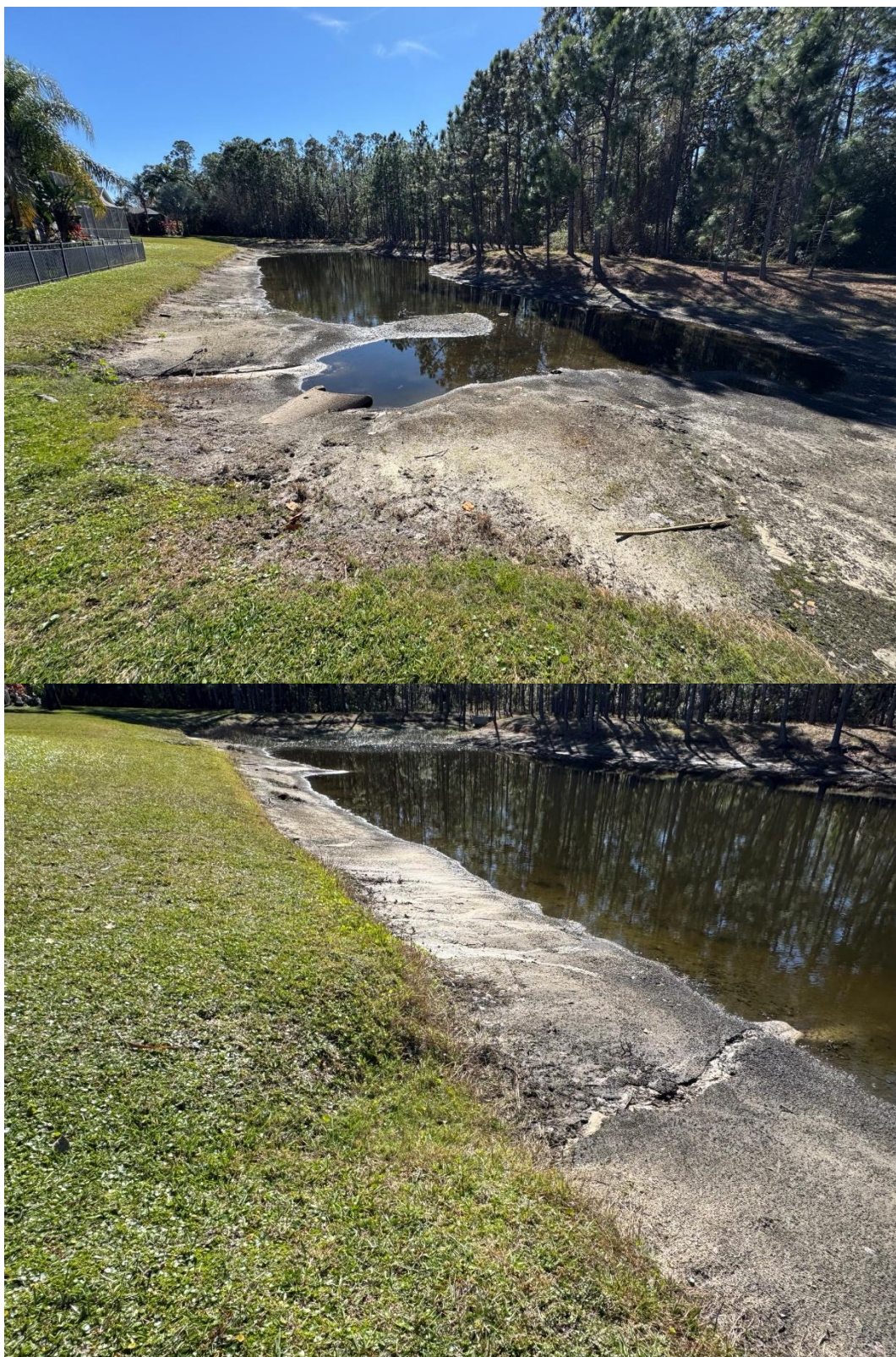
Photo 10 – Displays Pond 18 areas of pond bank erosion in the NE corner of the pond. Erosion appears to be caused by point sources from downspouts on the corner of the pond.
