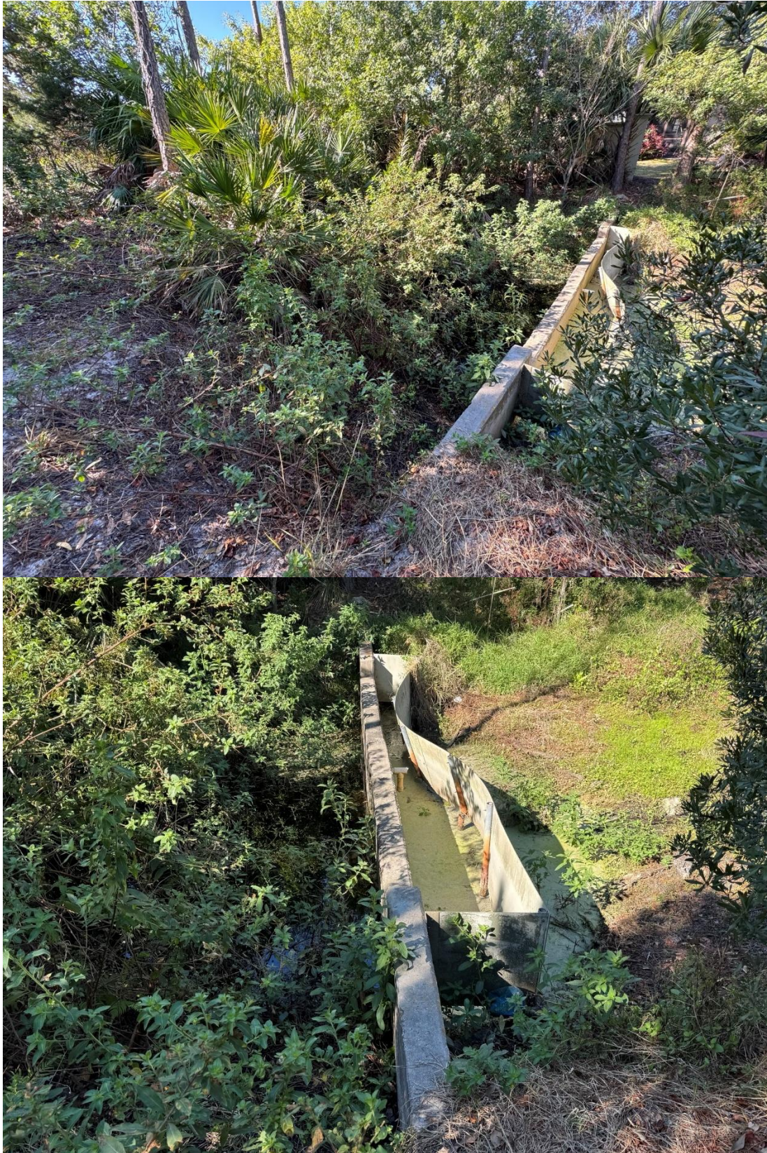
Photo 3 – Displays Pond 6 overgrowth on the back side of the weir structure and the broken skimmer (poles broken, skimmer blade still useable).
